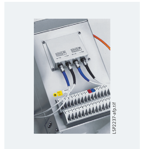
Fig. 5/93 Communication interfaces in a sloped case in a surface-mounting housing
